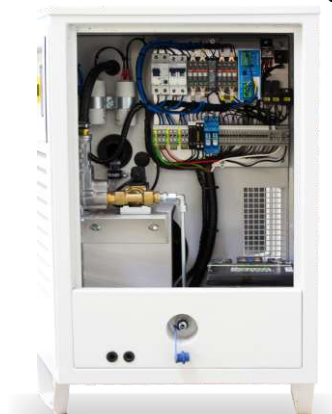
Integral emergency power supply
